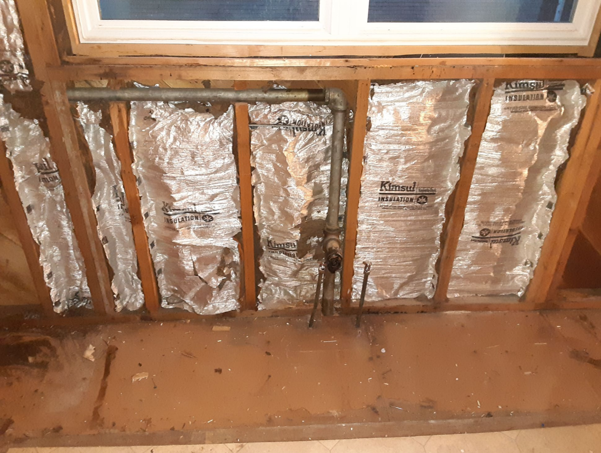
Outdated and insufficient insulation
