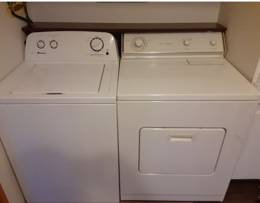
Re-plumbed the water lines and moved the washer from the opposite wall and placed next to the dryer
