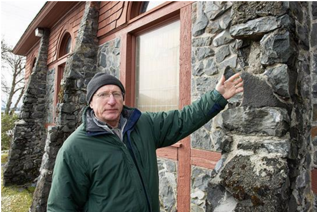
Loyd Platson, St. Peter's junior warden, recently points to stones in the church buttresses that are in need of re-pointing. (Sentinel Photo)
