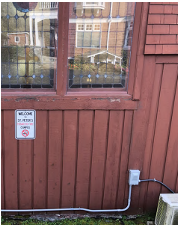
Figure 8.30: Original wall cladding below the timber datum has been replaced with T1-11 plywood siding.
