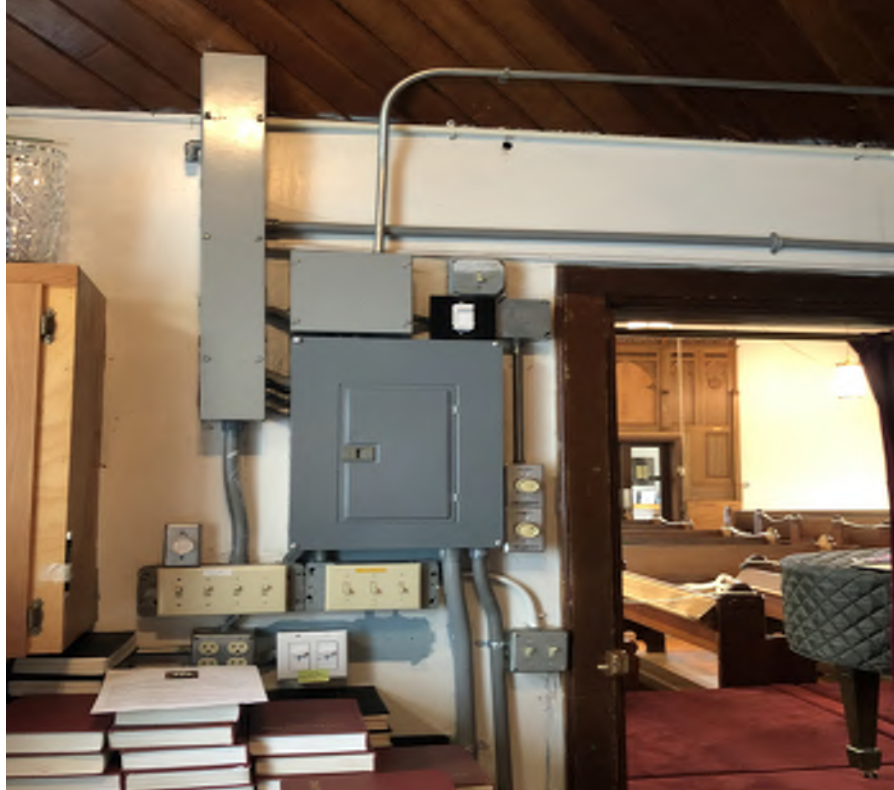
Figure 8.46: Electrical main distribution panel on kitchen wall.
