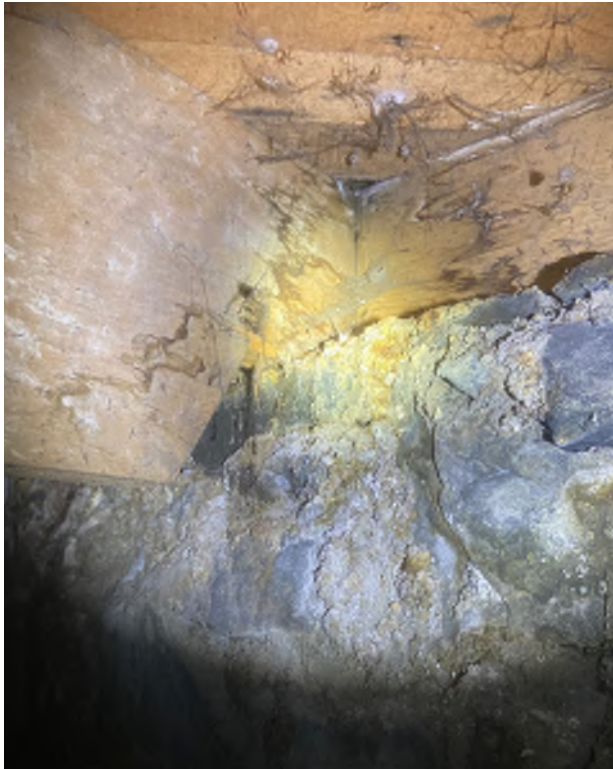
Figure 10.4: Wood rot visible at notch in floor joist. Photo credit: Sterling Holdorf
