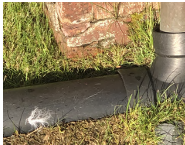
Figure 8.24: Several downspouts have black plastic pipe extensions attached to their lower ends, those located on the east transept discharge close to the building.
