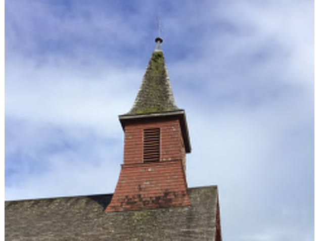
Figure 8.25: Heavy biological growth on the belfry roof, lower wall shingles, and the eaves and rakes of the main roof.
