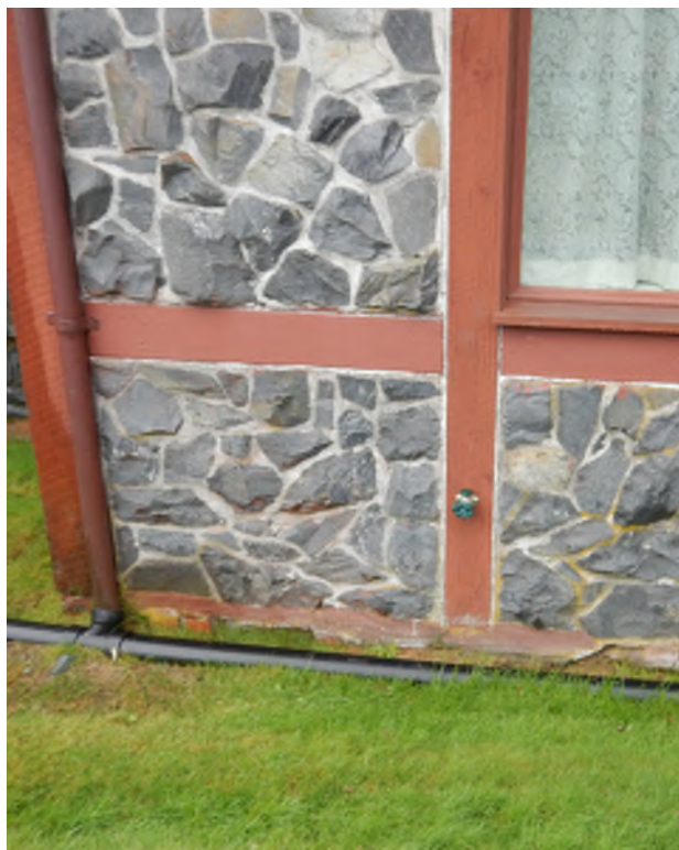
Figure 8.18: High soil levels on the exterior walls of the sacristy (east facade).
