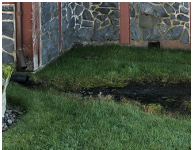
Figure 8.26: The downspout is disconnected at the northeast corner of the church, causing water to flow onto building walls.
