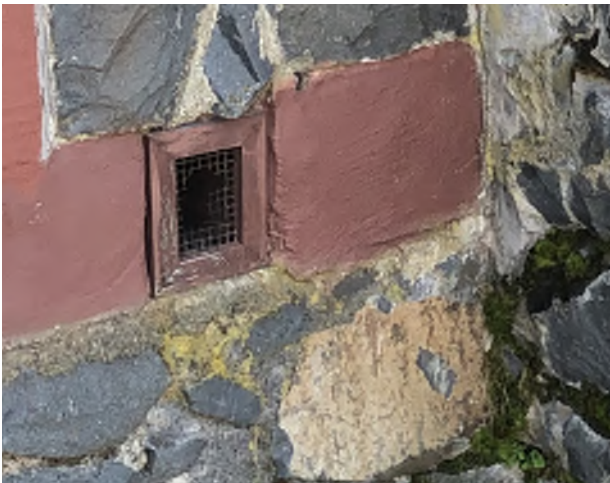
Figure 8.34: Damaged wire mesh on crawl space vent at the east facade.
