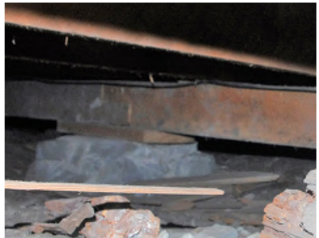
Figure 8.12: Flooring is supported by narrow beams at intermediate masonry foundation piers. Photo credit: Grant Crosby
