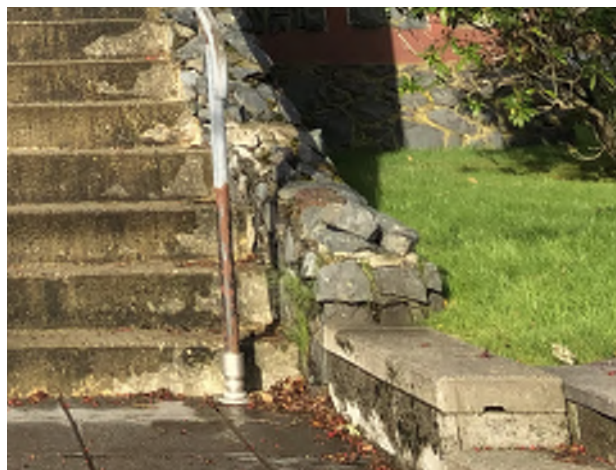
Figure 8.10: Loose stones and crumbling mortar caps on entrance stair walls are a falling hazard and potential tripping hazard.
