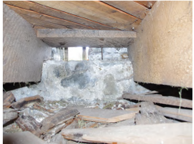
Figure 8.11: The wood floor structure consists of 2" by 11-7/8" solid sawn floor joists spaced 24" on center, cut at ends to rest on the brick leveling course. Photo credit: Grant Crosby
