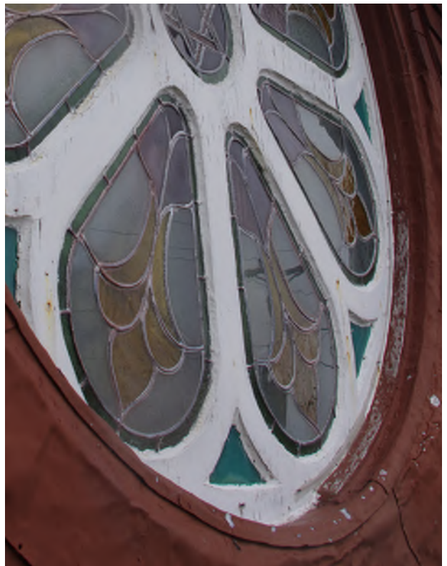
Figure 8.43: Weathered frame and muntins, and rust stains on the rose window located on the south facade.
