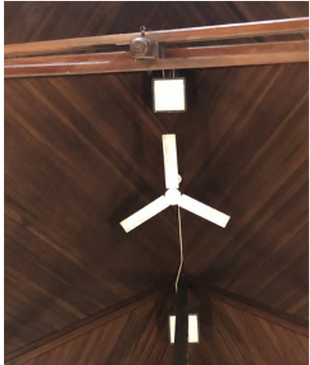
Figure 10.21: Paint ceiling fans in sanctuary to conceal appearance.
