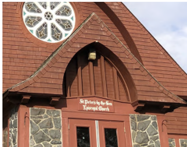
Figure 8.23: Soffits at the vestibule roof are supported by flat decorative corbels with an ogee profile not found elsewhere on the building.
