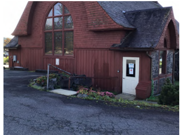
Figure 8.6: Secondary (rear) entrance on the north facade of the building is accessed from a combination concrete ramp and stairs.
