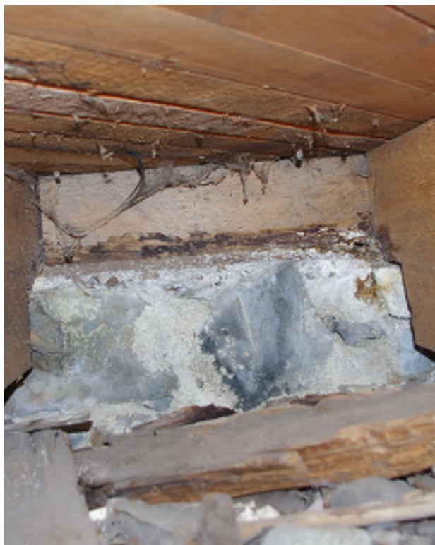
Figure 8.19: Visible debris between floor joists, minimal separation from soil, and decay at joist blocking. Photo credit: Grant Crosby
