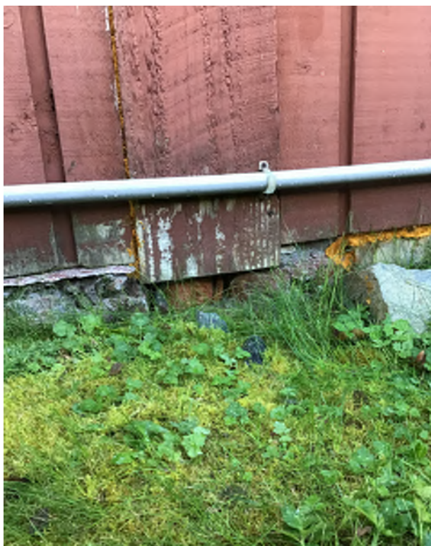
Figure 8.21: Spalling on parge coat, exposing mortar.
