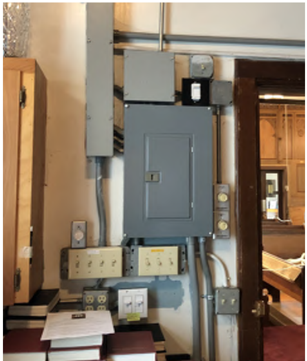
Figure 10.22: Hire qualified electrician to inspect electrical main distribution panel.
