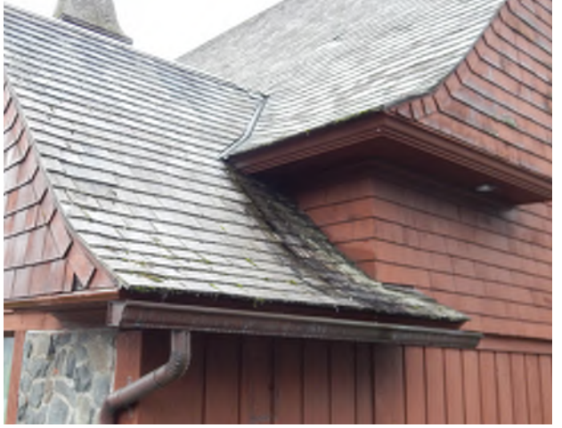
Figure 8.27: Metal flashing at the top of roof valley is poorly constructed and may not be properly directing water from the roof.
