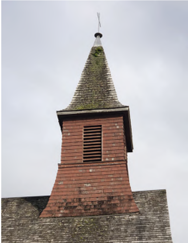
Figure 5.13: The belfry has vertically oriented, rectangular wood slat vents set within each of the four shingled walls.
