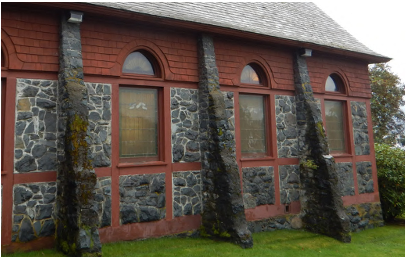
Figure 10.10: The repair and repointing of masonry buttresses is required due to prolonged water infiltration from roof runoff and repeated freeze-thaw cycles.
