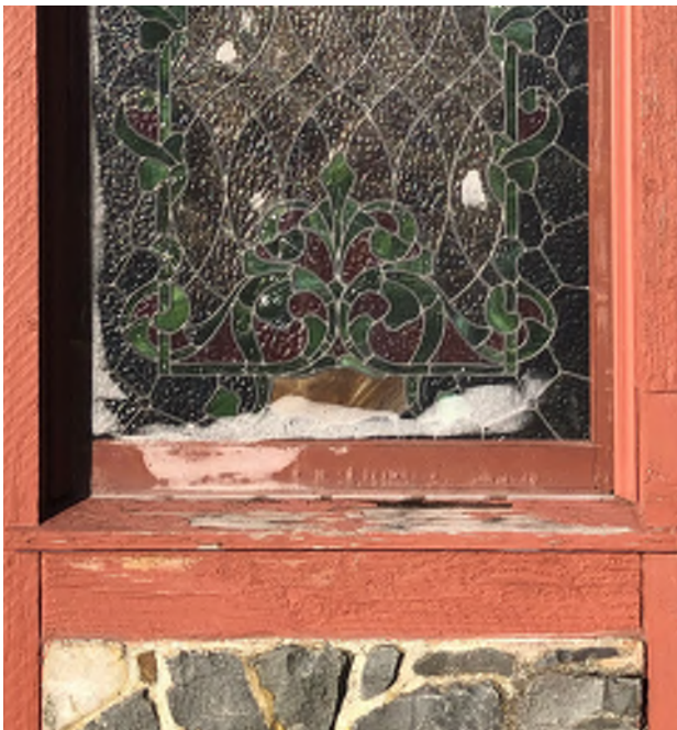
Figure 10.16: Remove failing paint and treat wood deterioration on wood sills on east facade.
