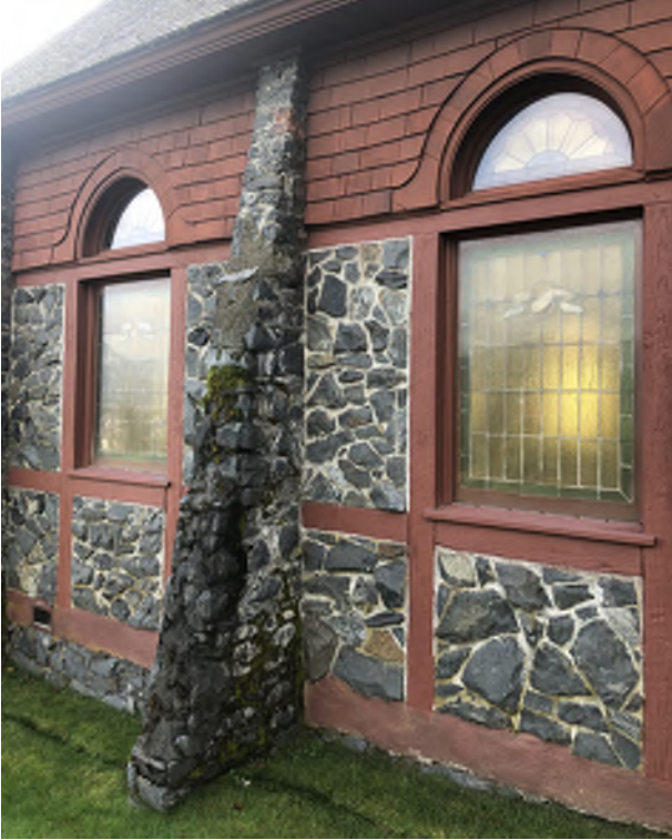
Figure 8.14: Buttresses span from the ground up to the underside of the roof soffit.
