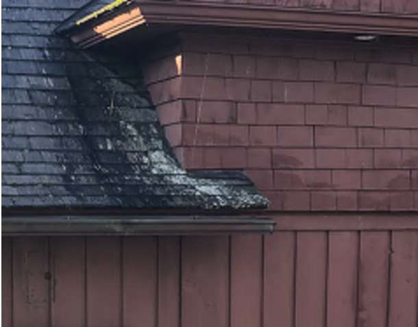
Figure 8.33: Shingles and plywood siding contain elevated moisture levels and evidence of biological growth.
