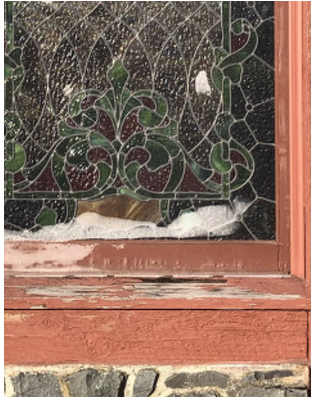
Figure 8.42: Visible deterioration on wood sill of windows on the east and north facades. Paint failure has caused wood to weather and be susceptible to moisture intrusion.
