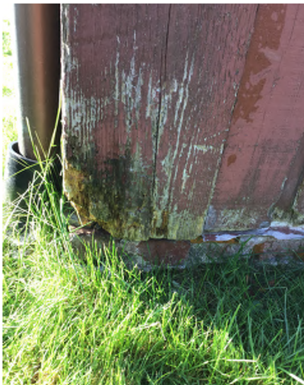
Figure 8.20: Rot deterioration and checking on half-timber framing column.
