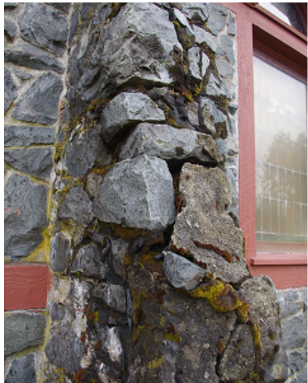
Figure 8.17: Cracks on the masonry mortar joints at the buttresses.
