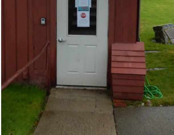
Figure 8.39: The north entrance door threshold exceeds the 1/2" maximum height and is not accessible.
