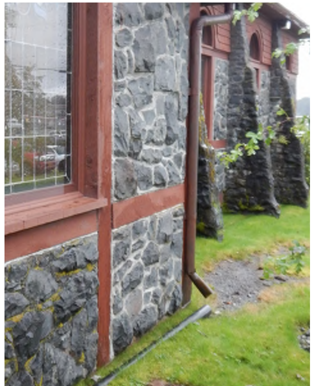
Figure 10.7: Reconnect joints in downspout at northeast corner.
