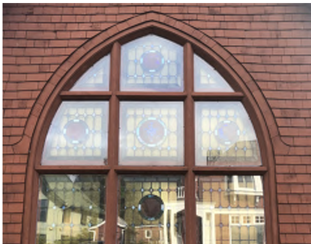
Figure 8.41: Divided stained-glass window on the north facade configured to match the hooded arches throughout the building.
