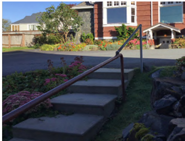
Figure 8.9: The pipe handrail serving the combination ramp/stairs at the north entry is not continuous and is lower than the required 34-38" height required by code.
