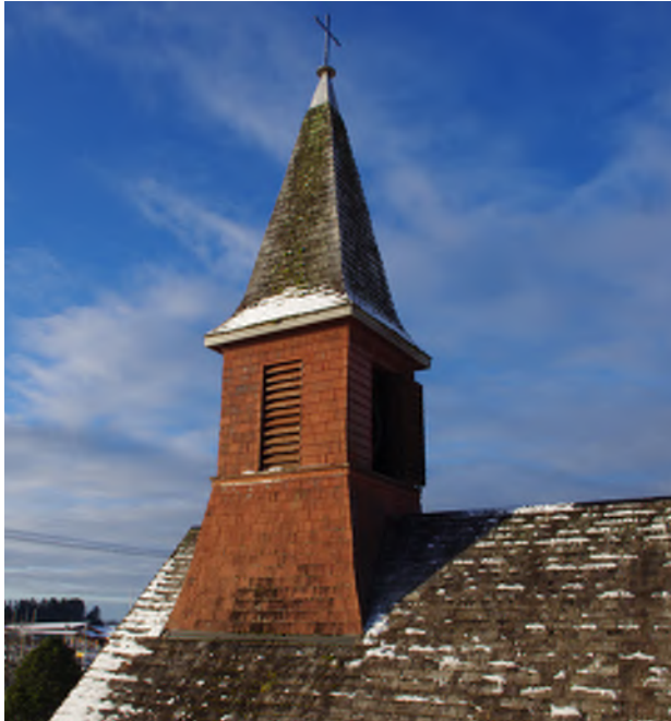
Figure 10.8: Provide cleaning, repair, and maintenance of belfry tower during next scheduled roofing campaign. Photo credit: Grant Crosby
