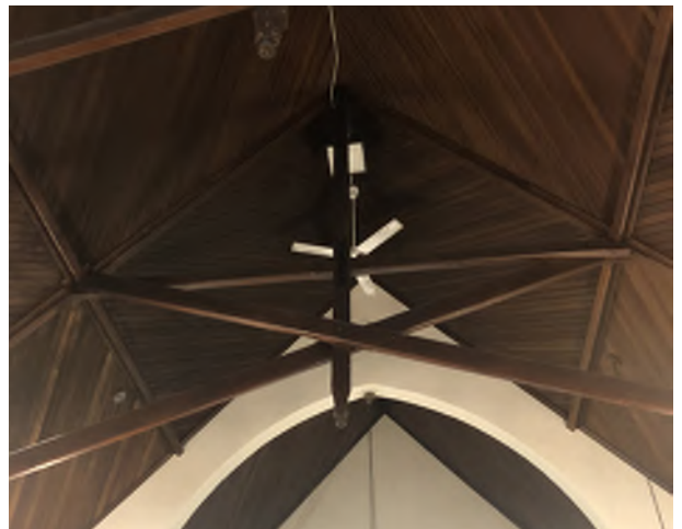
Figure 5.42: Detail of the diagonal tongue-and-groove dark wood beadboard ceiling, the scissor trusses and king posts with teardrop finials.
