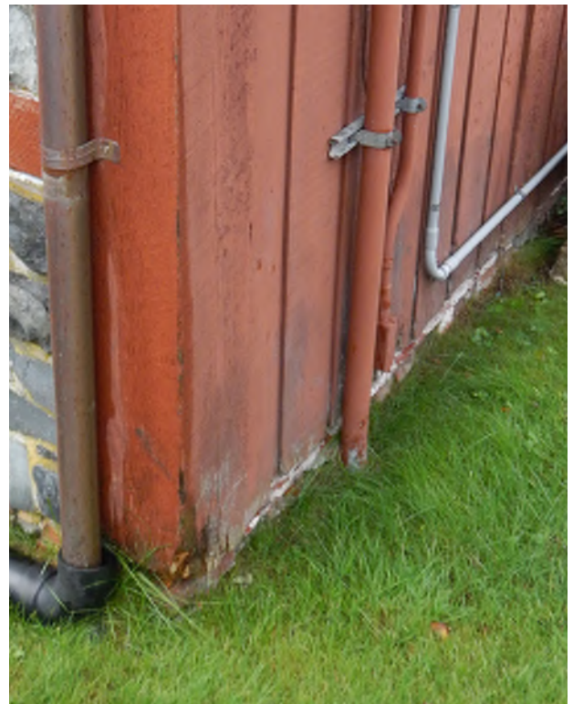
Figure 8.32: Evidence of wood decay at bottom edge of plywood siding on northeast corner of building.
