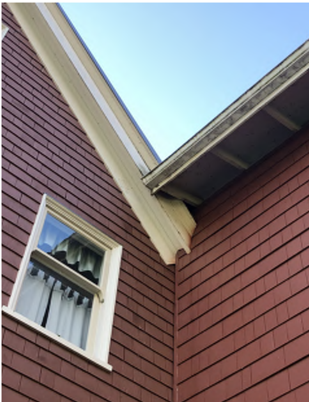
Figure 5.30: A detail of the intersection of the historic See House with the 1956 Fellowship Hall addition.
