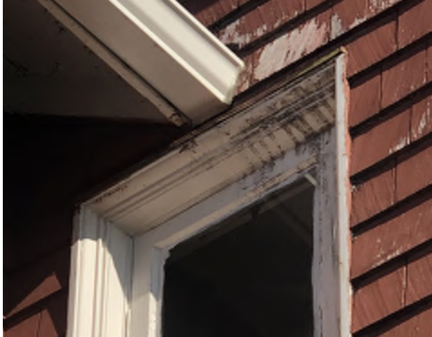
Figure 8.32: Staining on the upper casing and rail, with paint failure visible on the sill at Closet 205 window.
