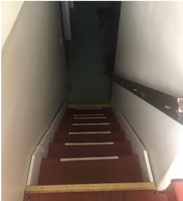
Figure 10.4: Provide code-compliant handrails at both sets of existing stairs to Basement.
