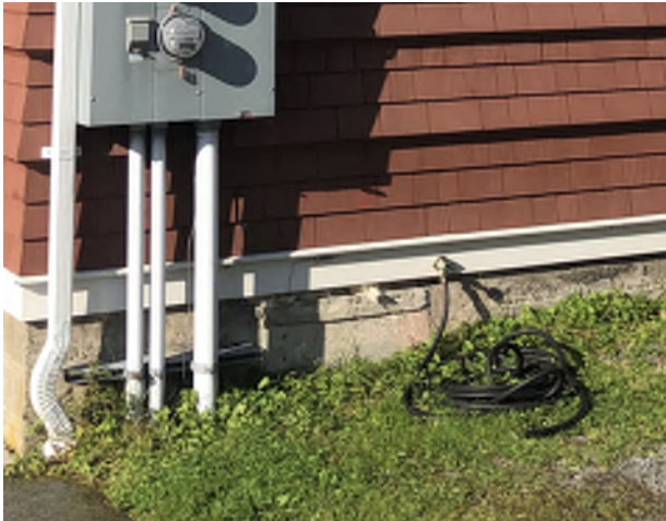
Figure 8.20: Water table on the east facade does not cover the foundation wall, exposing insulation and allowing an ingress path for rodents and pests.
