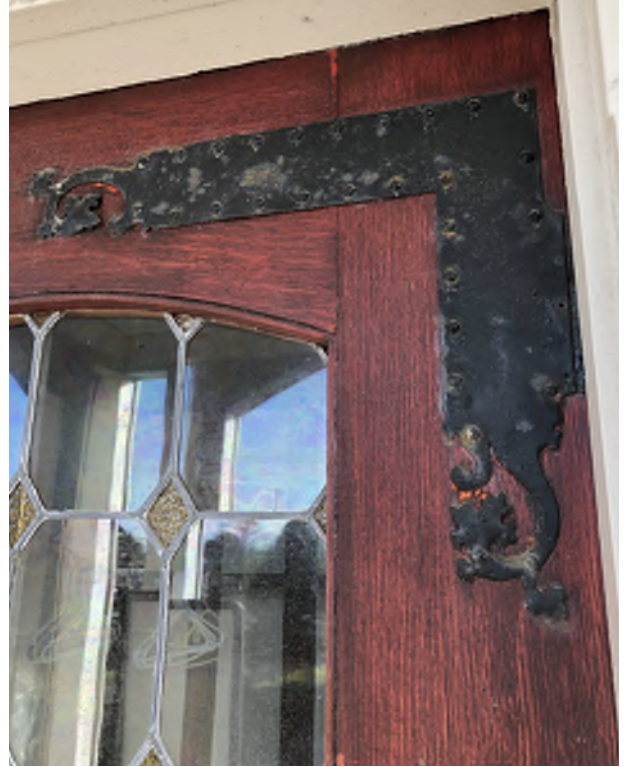
Figure 5.23: Detail of the leaded glass and metal decoration at the wood front door.
