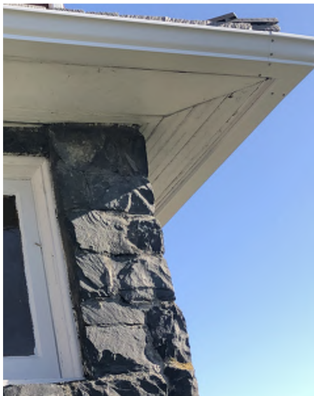
Figure 8.11: A majority of the original tongue-and-groove beadboard paneling on the eaves and soffits has been replaced with plywood.
