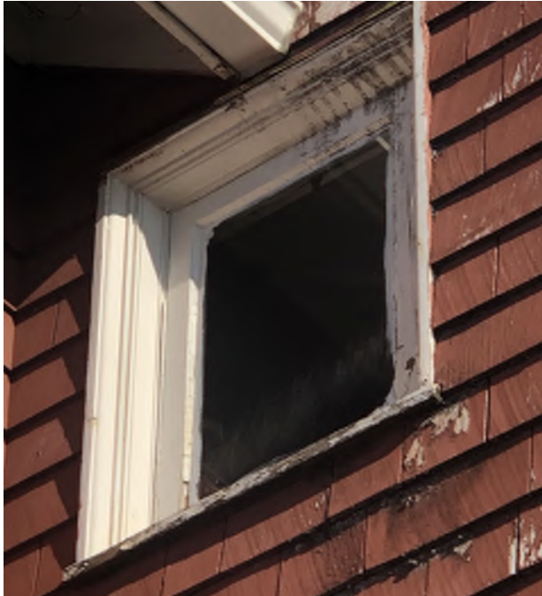
Figure 10.18: Inspect exterior and interior of Closet 205 window for wood decay and deterioration.
