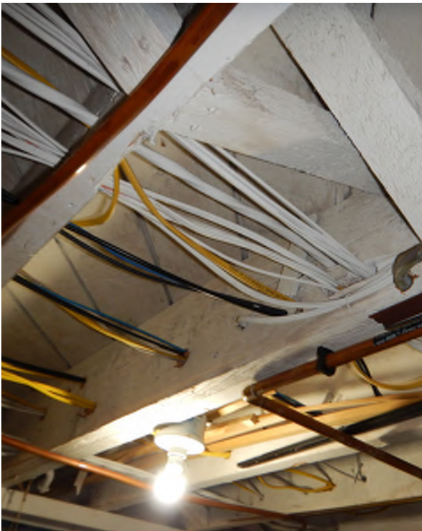
Figure 8.53: Overhead electrical wires and plumbing pipes.
