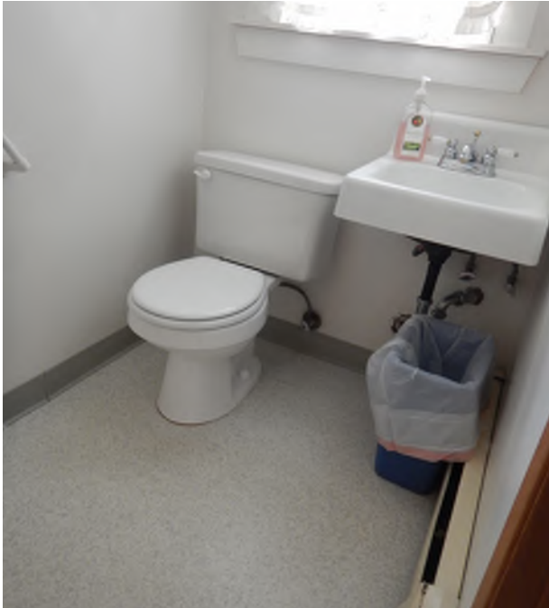
Figure 10.3: Install a code-compliant accessible restroom at Fellowship Hall.
