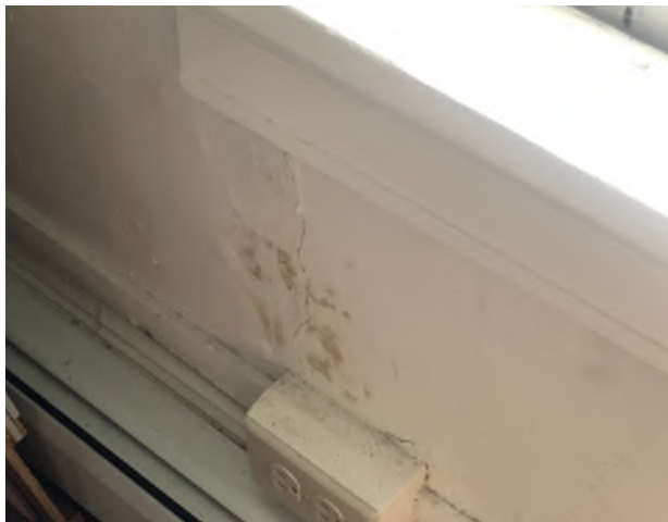
Figure 8.37: Damaged and cracked plaster below south facing window in Office 203 on the second level.
