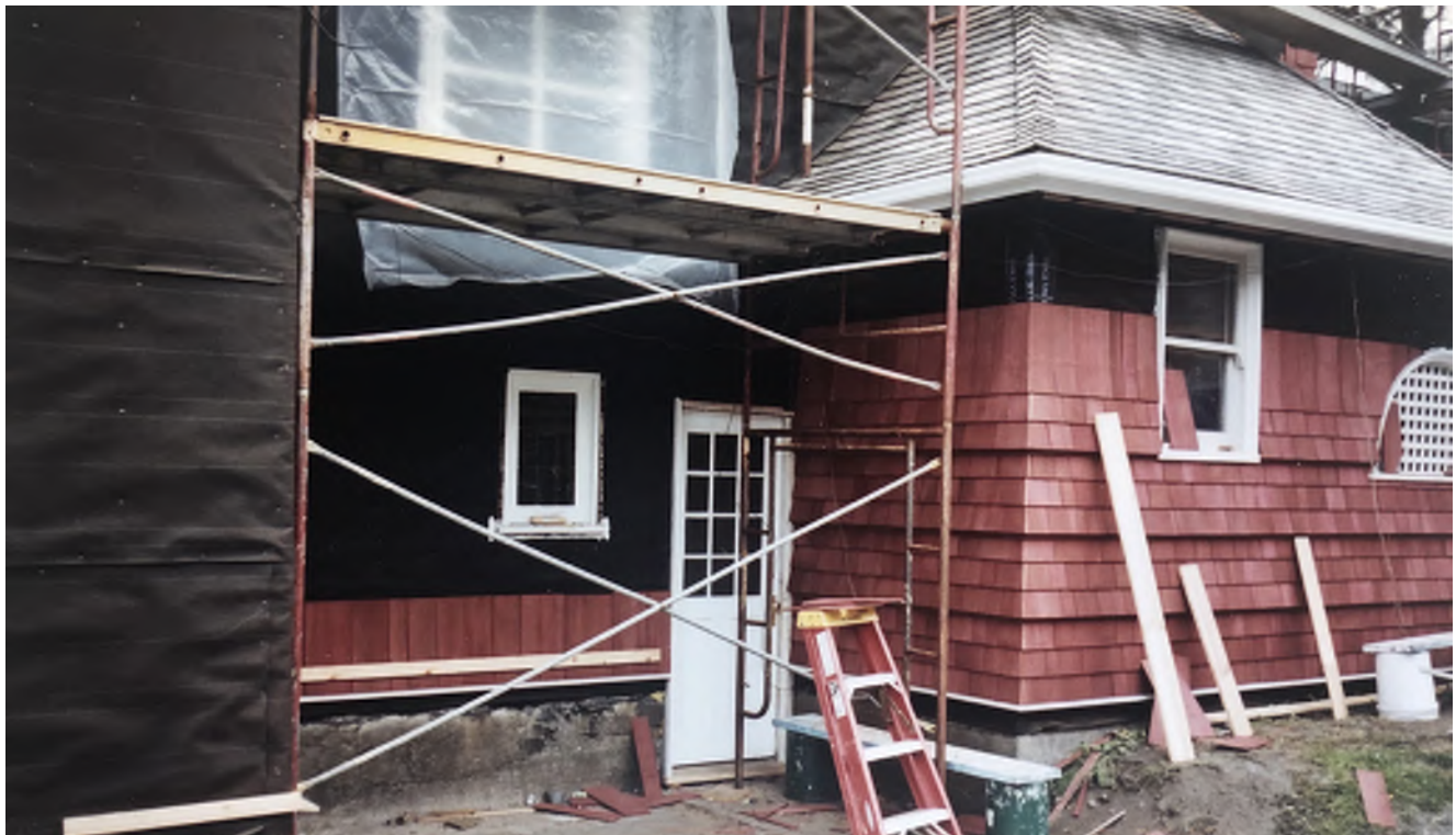
Figure 4.16: Photograph of 2003-2004 restoration of the See House. East facade showing installation of new shingles with underlayment paper installed, looking northwest. Source: St. Peter's by-the-Sea Archives.
