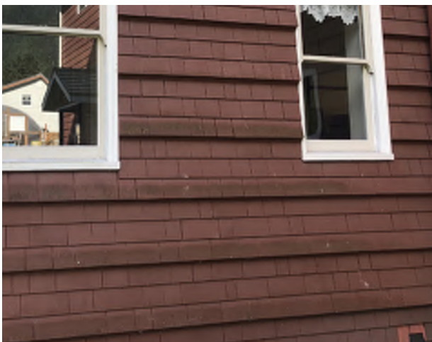
Figure 8.22: Mildew/soiling has accumulated on shingles, with highest concentrations on flared shingle course.
