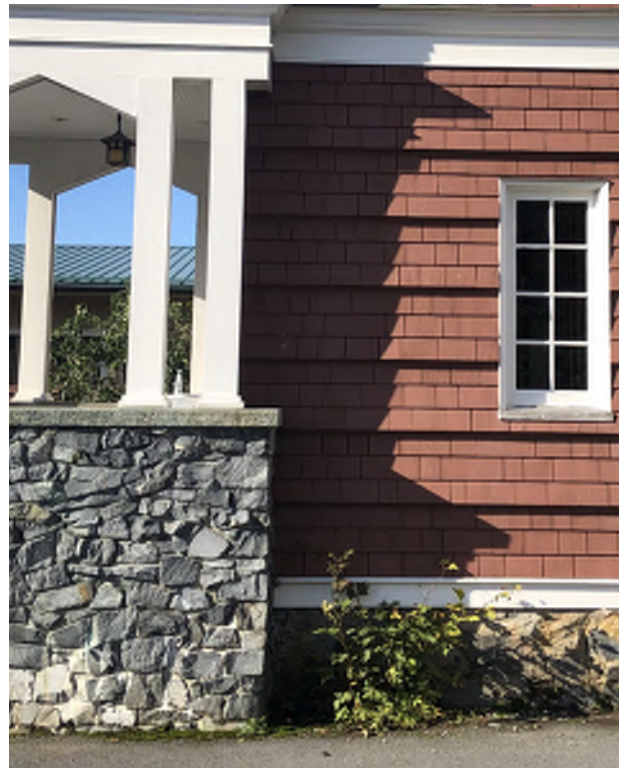
Figure 5.12: Exterior random laid stone at the stair and continuing to the foundation, which is partially obscured by landscaping, looking west.
