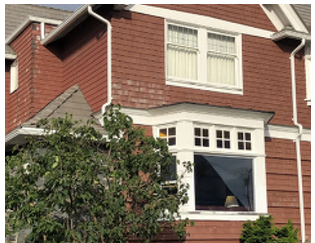
Figure 8.19: Weathered shingles on south (front) facade .
