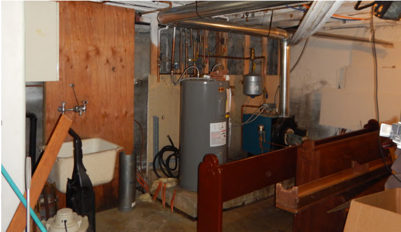
Figure 8.52: Mechanical heating system in the Boiler Room.
