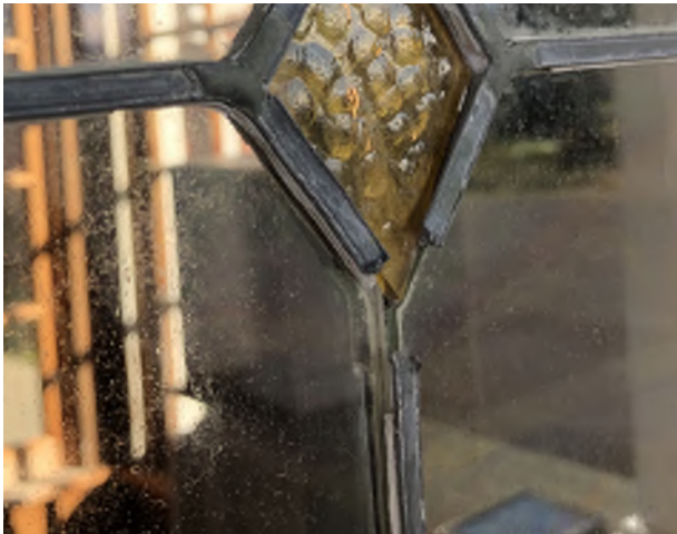
Figure 8.27: Deteriorated lead came at solder joints on the main entrance door leaded glass lite.
