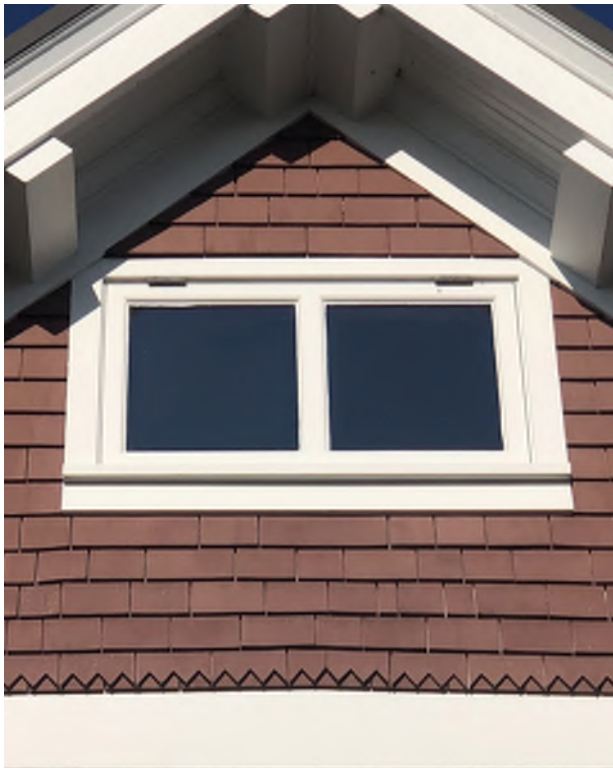
Figure 5.20: The front facing gable with the centered small awning window and decorative sawtooth shingles at the lower portion of the gable face.
