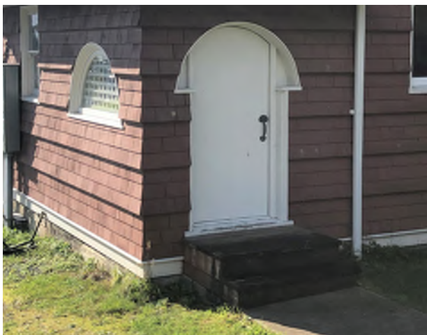
Figure 8.5: The north Kitchen entrance stairs are slippery when wet and pose a safety hazard.
