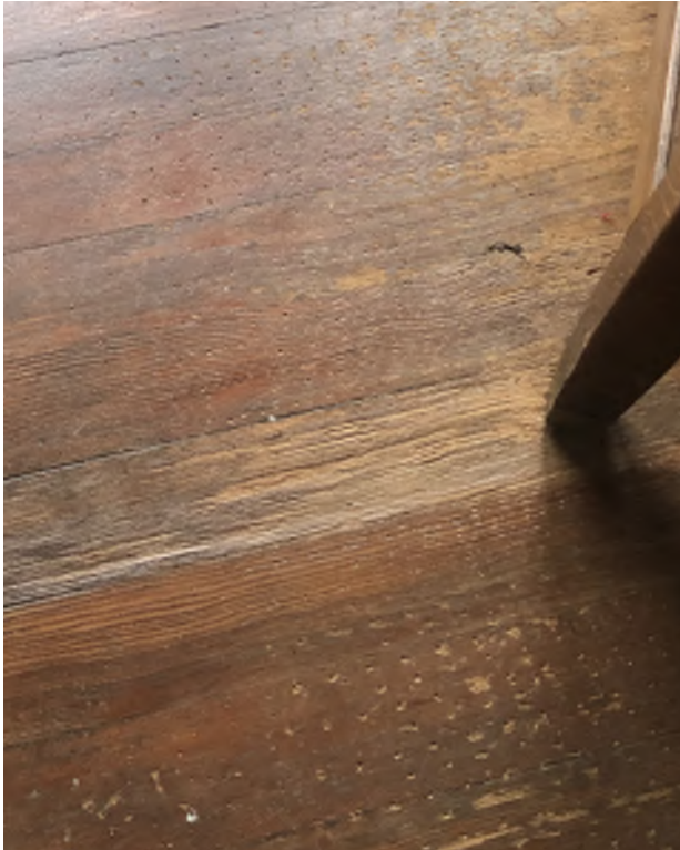
Figure 8.43: Worn and exposed surface of wood flooring in Office 203.
