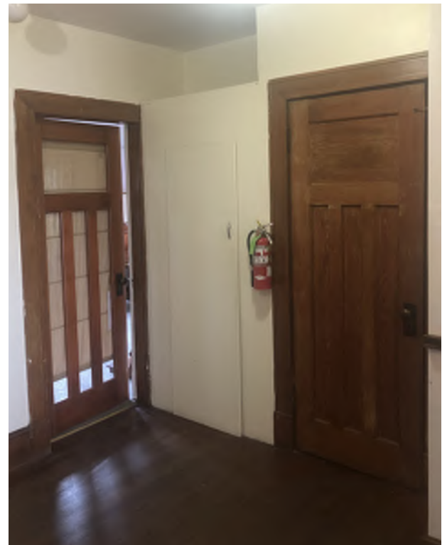
Figure 8.48: Uneven staining and discoloration on Attic door.
