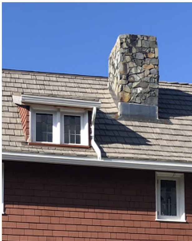
Figure 8.10: Unpainted wood trim at roof dormer on the east facade near the chimney.
