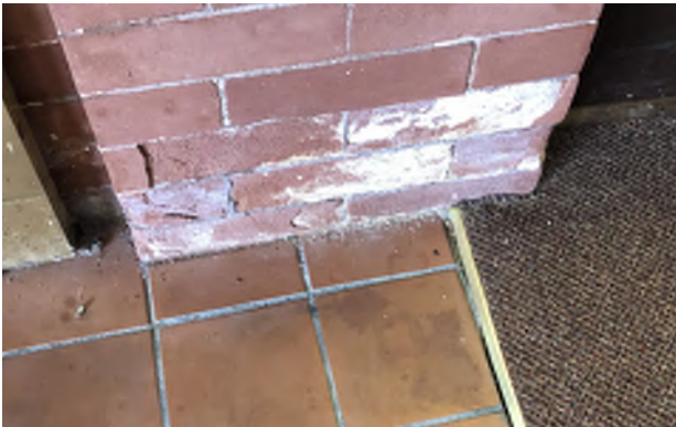
Figure 8.50: Evidence of deterioration and spalling of brick surface, and damaged tile grout.
