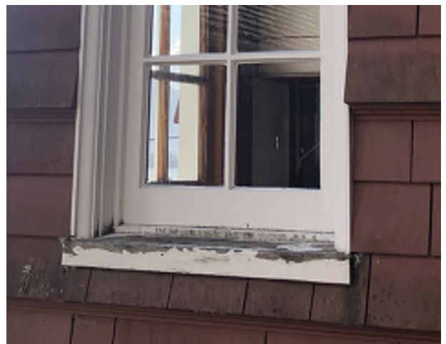
Figure 8.31: Paint failure on east Entry Vestibule window.
