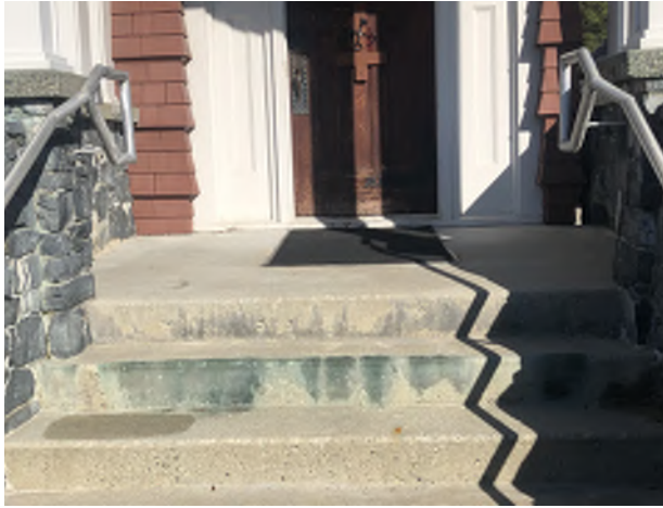
Figure 10.14: Green staining from oxidization and runoff of copper flashing above entry stairs.
