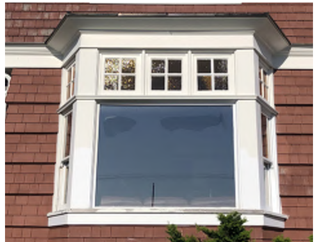
Figure 5.17: Detail of the lower story bay window on the south façade, looking north.
