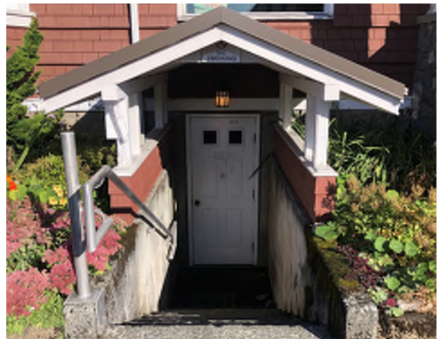
Figure 8.24: Basement entrance (a later addition) cut into concrete foundation walls, accessed from concrete stairs.
