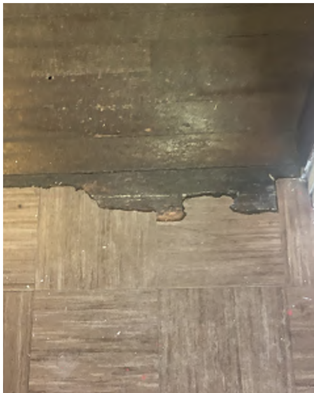
Figure 8.44: Damaged floor tiles at door threshold of Father's Study.
