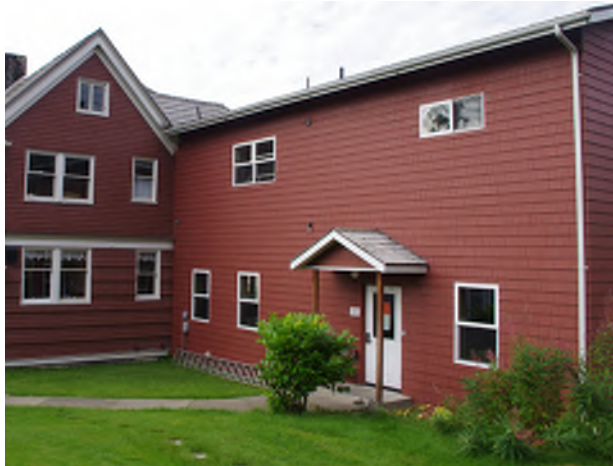
Figure 10.8: Add additional downspouts to See House and Fellowship Hall. Photo credit: Grant Crosby
