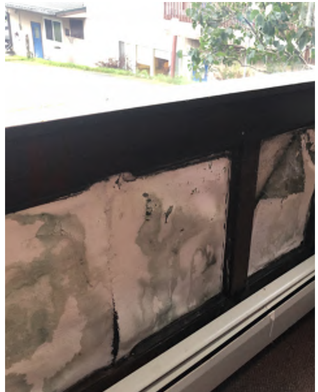
Figure 8.35: Plaster and burlap wall panel coverings in poor condition on the interior wall beneath the bay window in the Living Room.
