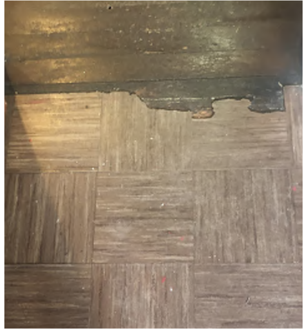
Figure 10.24: Contact certified inspector to have tile flooring in Father's Study tested for asbestos.
