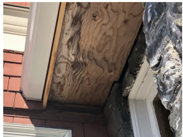
Figure 10.12: Replace plywood with tongue-and-groove beadboard at soffits.
