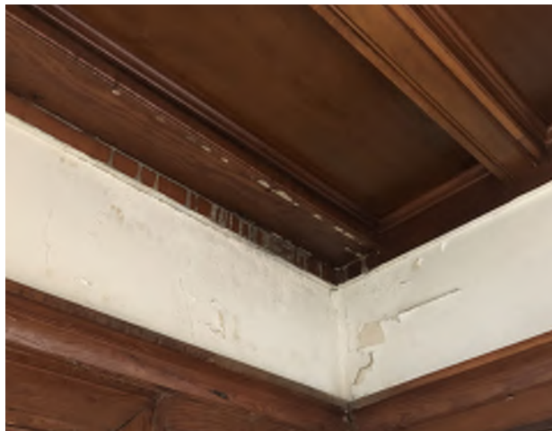
Figure 8.40: Water damage on ceiling and walls in Entry Vestibule.
