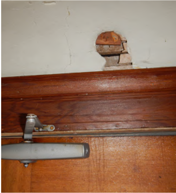
Figure 10.22: Restore deteriorated plaster wall finishes on first and second floors.
