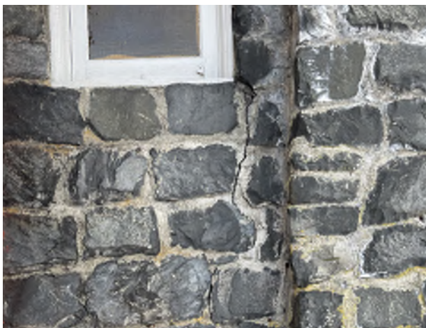
Figure 10.15: Repair vertical mortar joint crack at north side of chimney. Photo credit: Troy Feller
