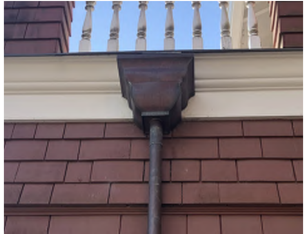
Figure 8.12: Copper leader and round downspout on the east of the entry porch balcony.
