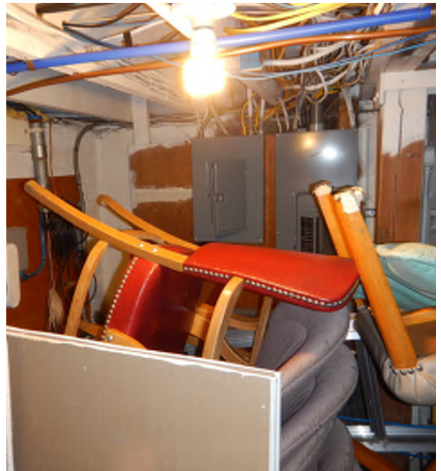
Figure 10.29: Remove material stored in Boiler Room to provide a clear pathway and code required access to mechanical equipment and electrical panels.
