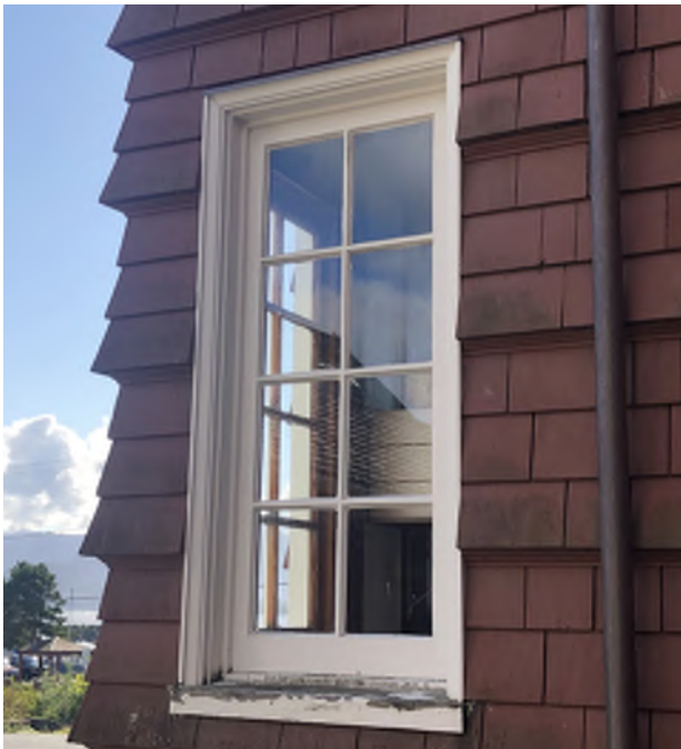
Figure 10.19: Remove failing paint from deteriorated wood sills and repaint to protect wood.
