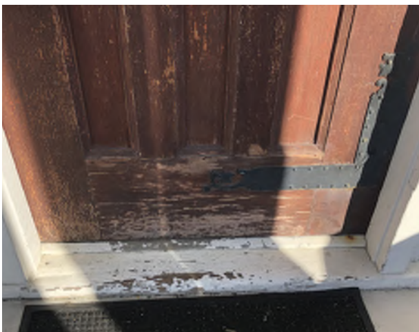
Figure 8.28: Stain finish of main entrance is in poor condition due to general wear and tear and lack of stain maintenance.
