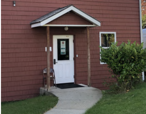
Figure 8.3: The landing outside of the Fellowship Hall entrance does not have a code-compliant clear floor area.
