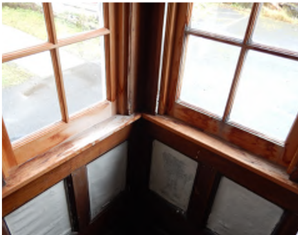
Figure 8.33: Interior moisture damage visible on the interior of sills at southeast Entry Vestibule windows.
