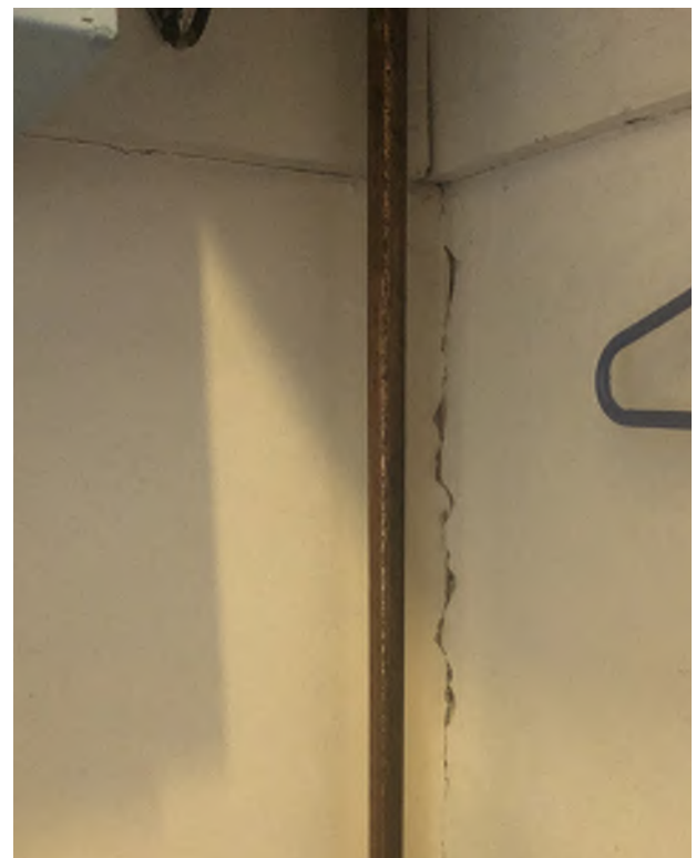
Figure 8.36: Significant crack in plaster wall next to copper pipe in Storage 204.
