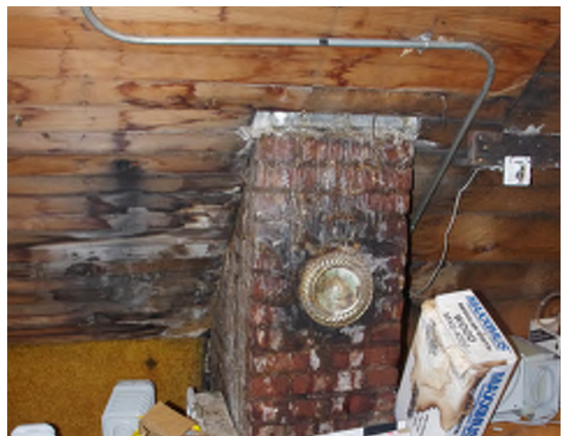
Figure 8.7: Moisture infiltration at the attic level around the Boiler Room chimney.
