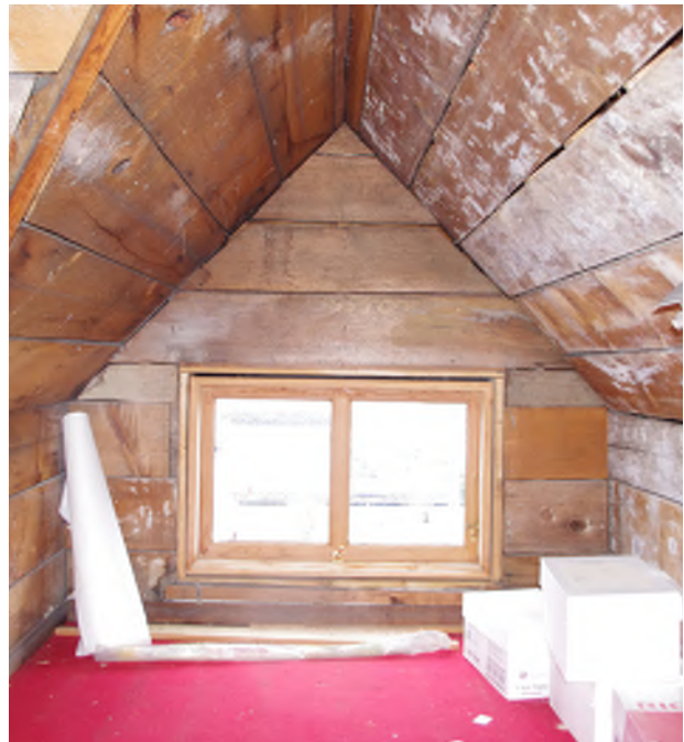
Figure 10.21: Remove mildew from all wood surfaces in Attic. Photo credit: Grant Crosby
