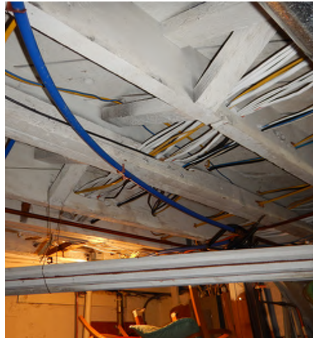
Figure 10.6: First floor joists should be evaluated by a structural engineer.
