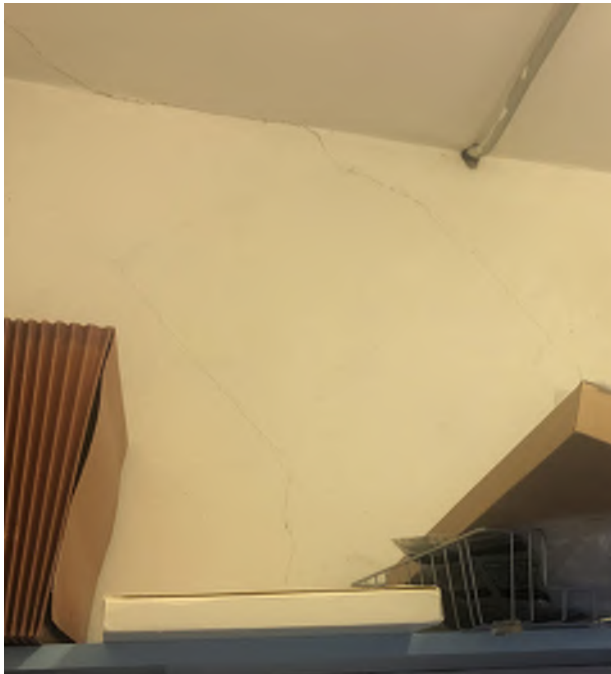
Figure 10.23: Repair hairline cracks and repaint ceiling finishes in storage closets on second floor.
