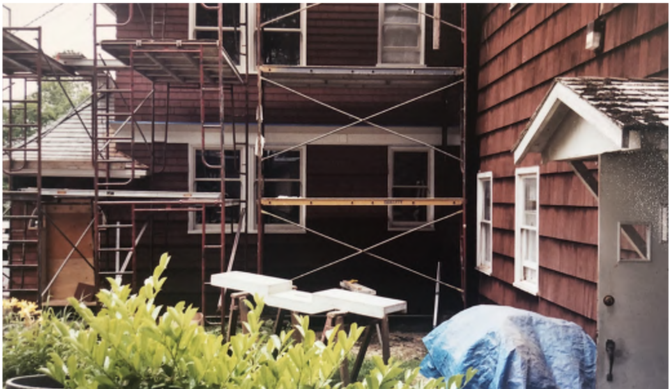
Figure 4.17: Photograph of 2003-2004 restoration of the See House, installation of shingles and repair of doors and windows on the north facade of the See House, looking south. Source: St. Peter's by-the-Sea Archives.
