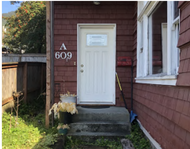
Figure 8.4: All entrances (with the exception of the main entry) are not code compliant due to the absence of handrails and/or handrails on both sides of stairs.
