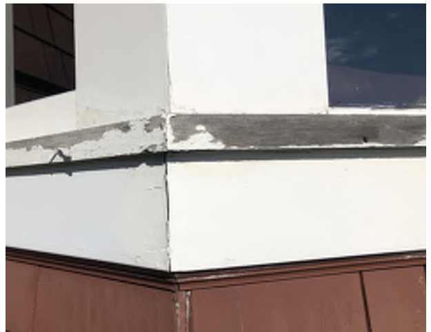
Figure 8.30: Weathered and deteriorated window sill on south bay window.
