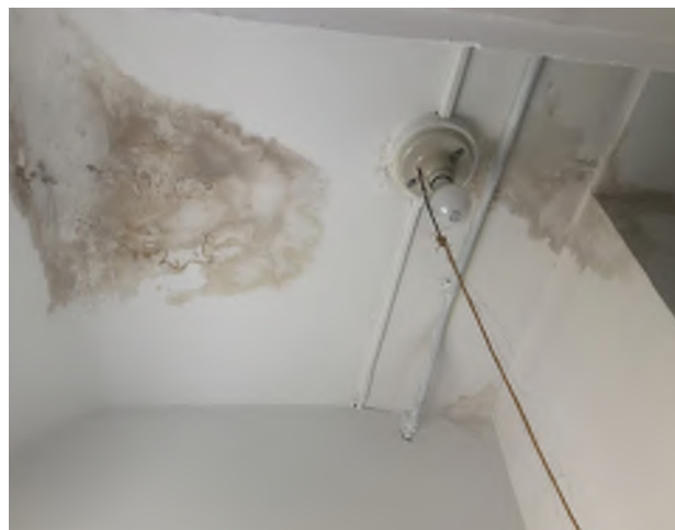
Figure 8.41: Moisture stains on plaster ceiling in Closet 210.
