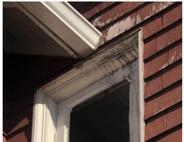
Figure 8.13: Inconvenient placement of the gutter above the window located on the west facade at the Bishop's Closet.
