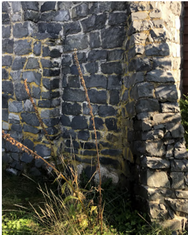
Figure 8.16: Stone masonry buttress is in poor condition and efflorescence and moss growth are visible on masonry.
