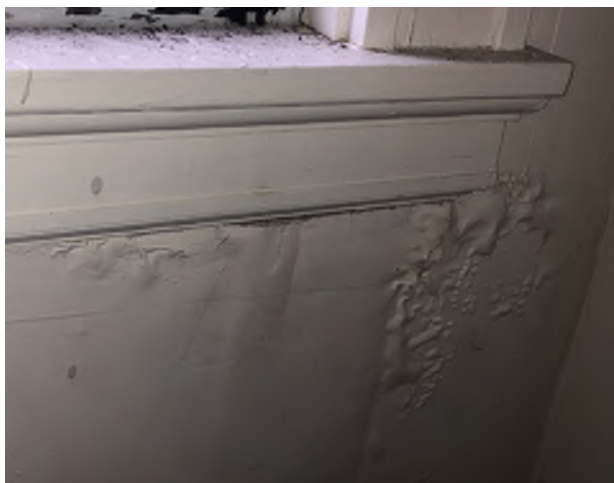
Figure 8.38: Moisture intrusion related to exterior gutters has delaminated and cracked plaster walls below the window sill of Closet 205.
