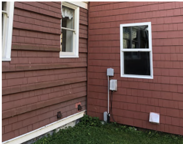
Figure 8.21: Exterior of addition lacks a water table at the base of the shingle siding.
