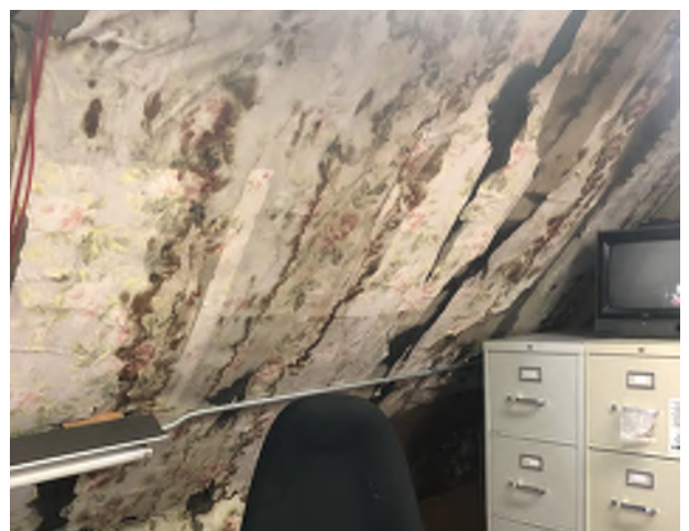
Figure 8.14: Peeling wallpaper in Attic due to elevated levels of humidity and moisture on wood substrate.
