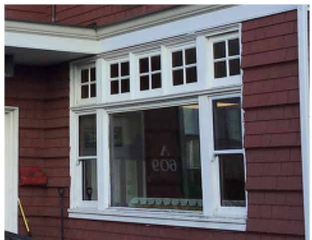
Figure 8.8: Slight sagging of window head on the exterior of the Dining Room window on the west .
